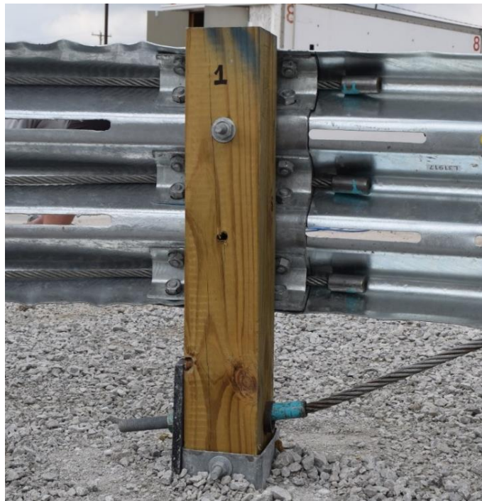
Figure 29. Nose Cable Attachment at Post 1
